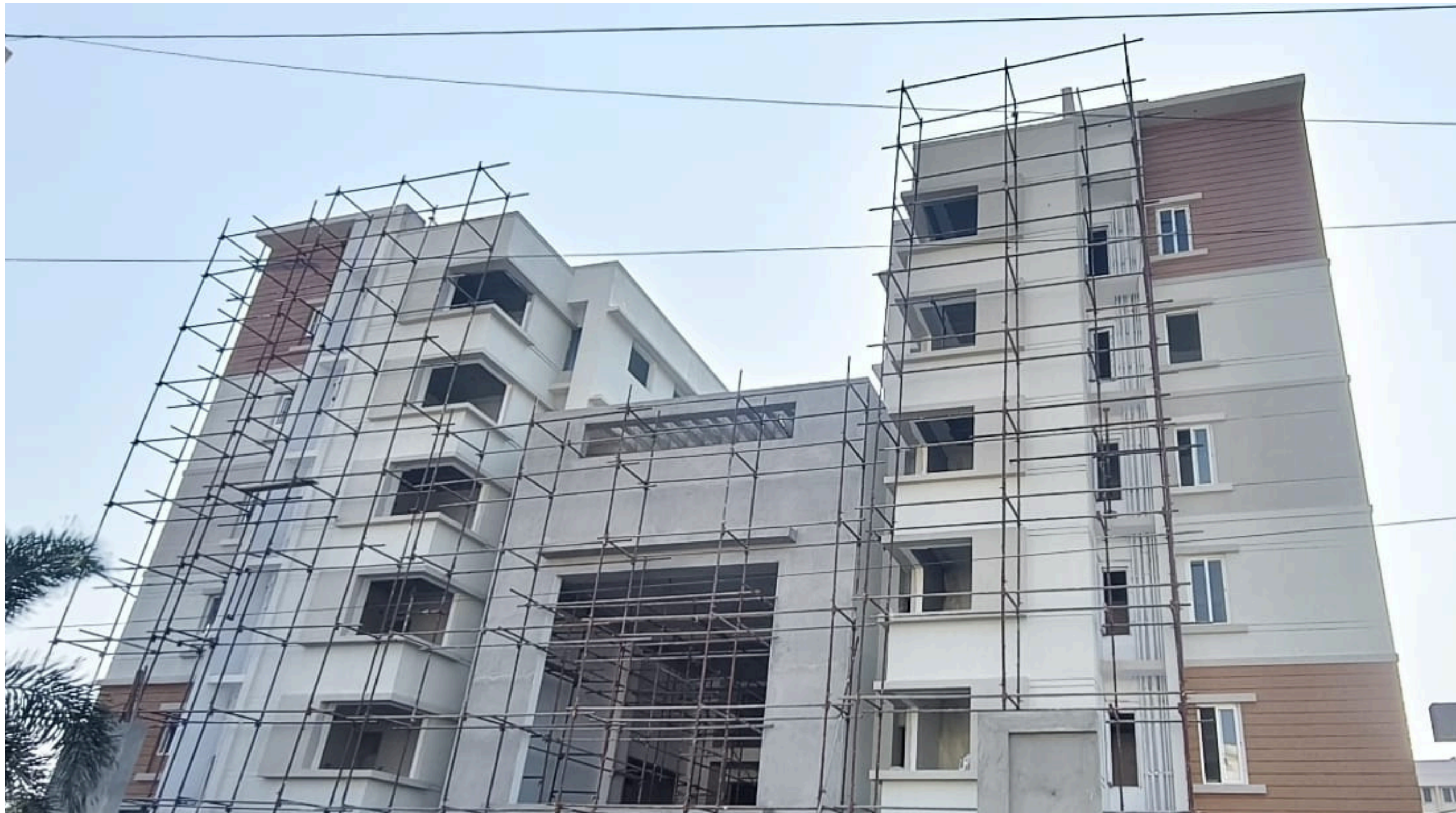
Main Building East Side External Texture Painting 1 st Coat Work In Progress.
